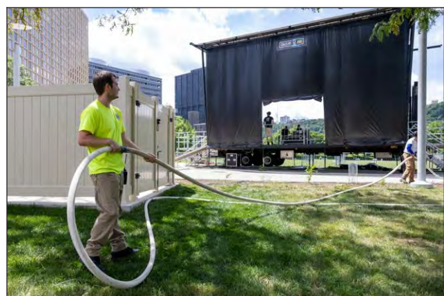
Crews build the stage at Point State Park. The festivities begin Friday and continue through Sunday.
