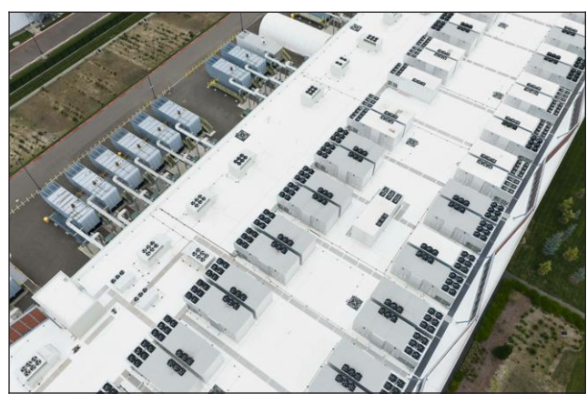
Fans, part of a cooling system, are visible on the roof of a data center in Hillsboro, Ore.
